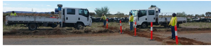
The Alice Springs Correctional Centre, Community Support Work Party assisting with laying a camera cable for the Finke Desert Race, June 2016
