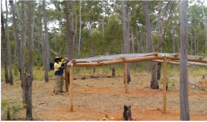
A new shelter being built by prisoners from the Datjala Work Camp for the women to meet and sleep at the Garma Festival.
